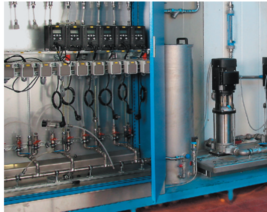
The DME dosing pumps at Wisthoff Glassworks in Germany.
